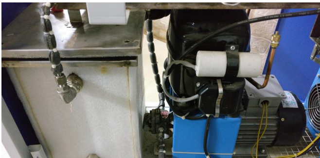
Figure 9 Compressor Refrigeration System
